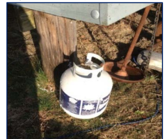
Unsafe propane storage. (2 photos below)
