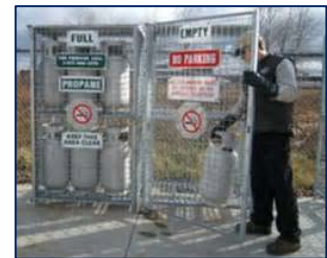
Safe propane storage in cage with signage. (photo above)
